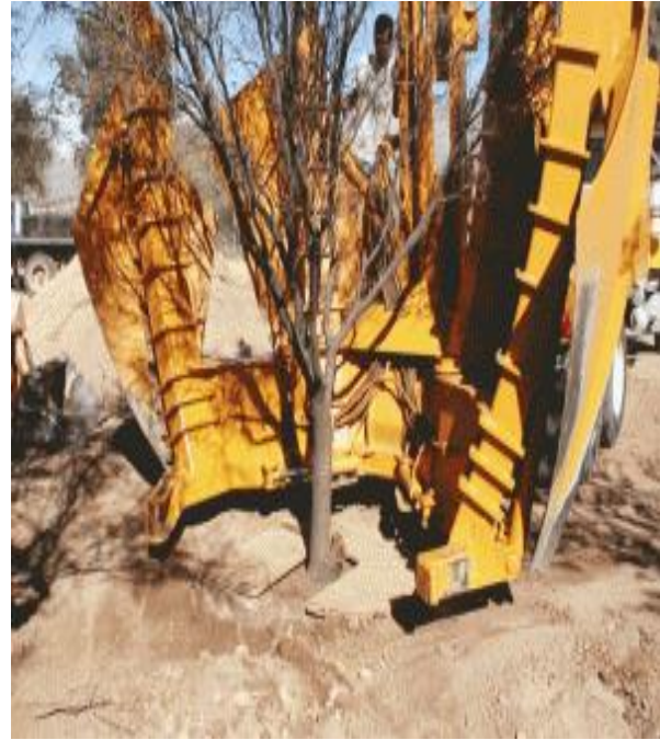
It is then moved to the donor location and positioned with its blades raised and the gate open around the tree
